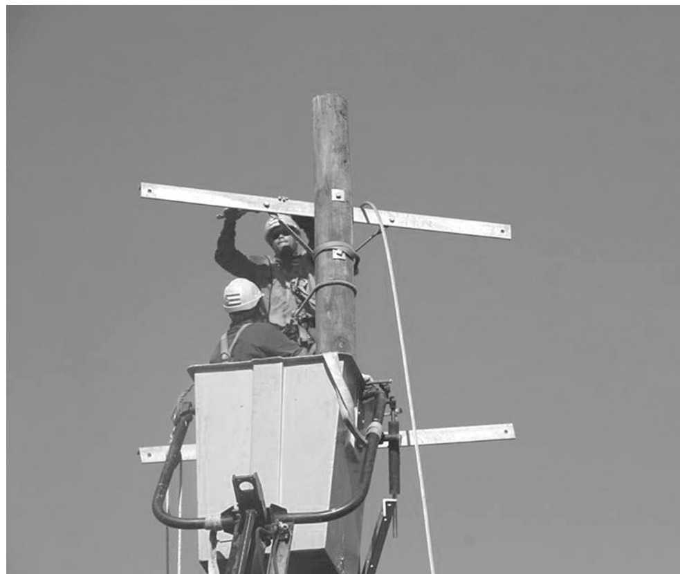
Cuban specialists are working on a primary line linking the capital with the hydroelectric plant in Trafalgar, eight kilometers away.
